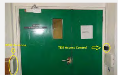
Figure 3: Installation at CEE 1.09 Computer Lab
