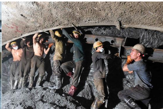
Fig. 4 – A group of workers lacks protection
