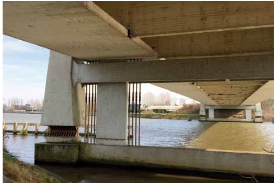
Fig. 12 Lower part of one of the piers of bridge W16 (Photo: Luc Taerwe)
