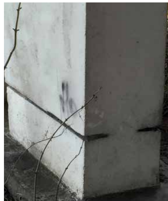
Fig. 5 Freyssinet hinge at lower part of V-shaped bearing wall (Photo: Luc Taerwe)
