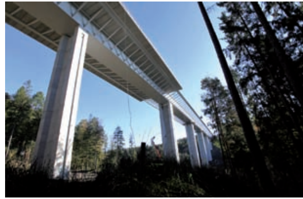
Fig. 16: Progressive assembly of the deck of the Bridge across the Kremlice Creek Valley (Photo: Jiri Dvorak)
