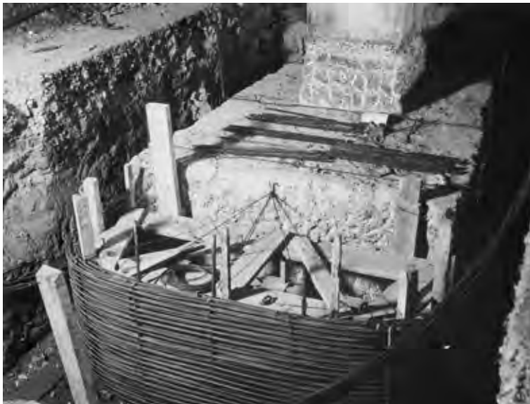
Figure 36 Anchor blocks at the Maritime Station of Le Havre, solution for rehabilitation by Freyssinet in 1934
