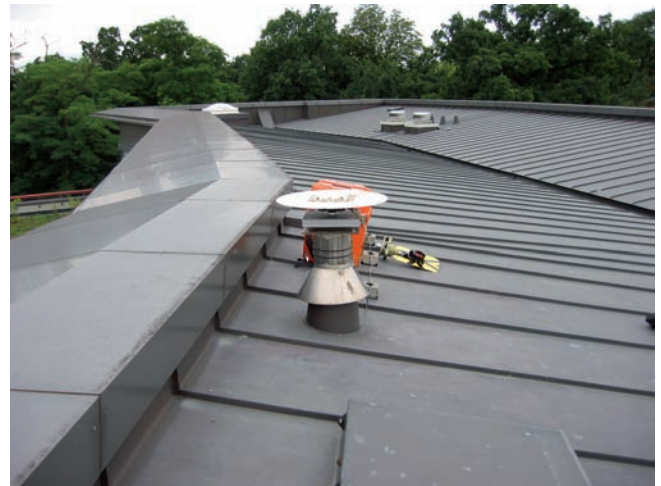
Figure 6. Detail picture of the station surrounding of CORS 0078 (facing west) before the change to a choke ring antenna. The balustrade on the left causes false carrier phase multipath estimation.
