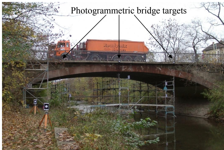
Figure 8: Franckebrücke at Erfurt with the trestle for fixing the inductive gauging sensors, the targets for the photogrammetric measurement and the trucks
