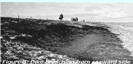
Figure 3: Dike breaching from seaward side
