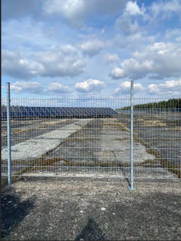
LEAG's Solarpark Welzow III
