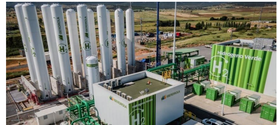
Puertollano Green Hydrogen Plant, Spain [8]
