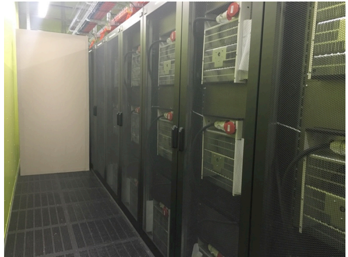
Fig. 4 Test room with screen for thermal imaging (left) and racks with air heaters (right)
